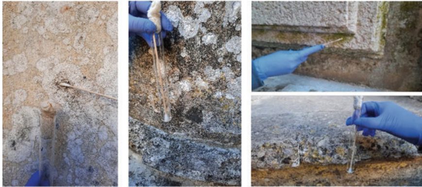
Fig. 10.2 Sample collection from various pigmented biofilms formed on the limestone walls of the Main Cloister
